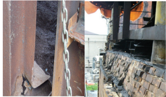
New construction does not have support columns like this or beam flanges supported by bricks
