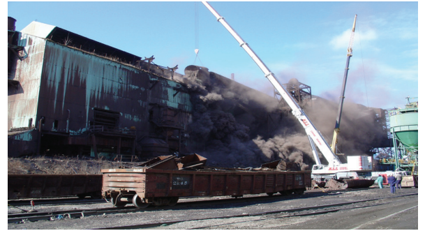
What if there is a surprise Inside the pipe you are cutting?
