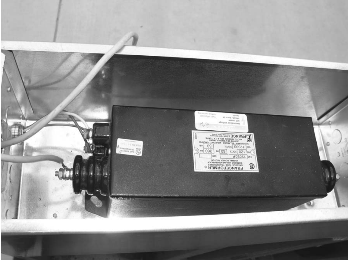
Figure 6 - Non-self contained neon transformer in metal box
