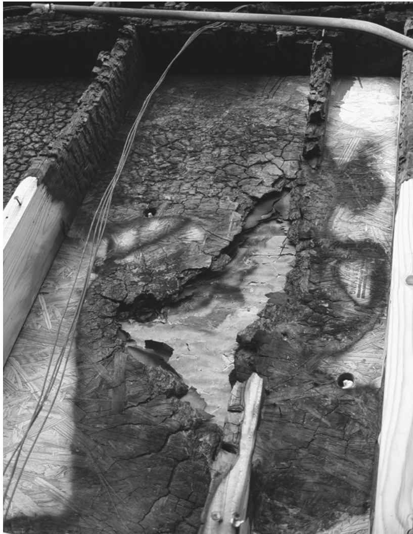
Figure 2 - Stucco scorching inside at point of origin
