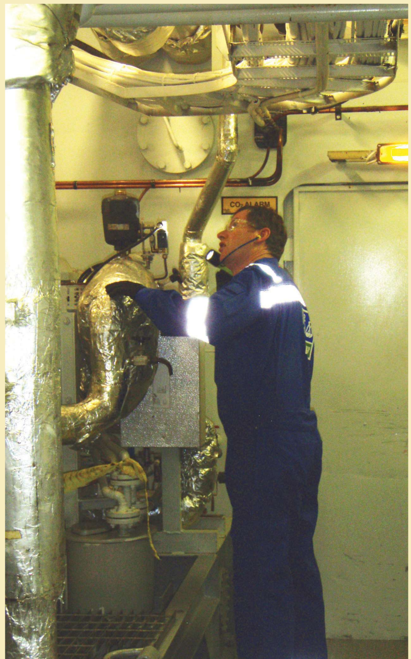
A surveyor witnesses fuel pump remote shutdown.
